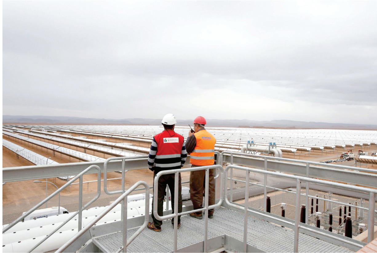
A thermosolar power plant at Noor II Ouarzazate, Morocco.
